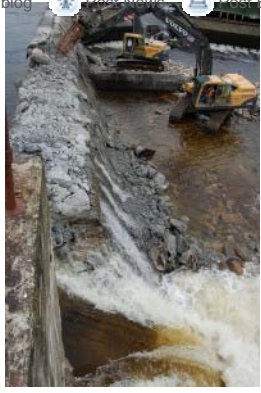
Water flows through the Great Works Dam after it was breached. Photo courtesy of the Penobscot River Restoration Trust
