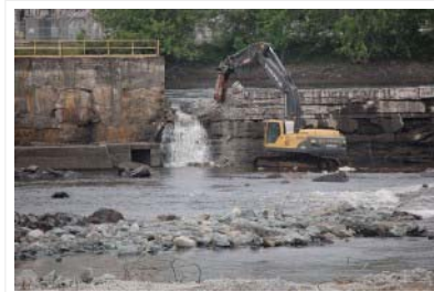
Work crews breached the Great Works Dam in Bradley on Saturday. Photo courtesy of the Penobscot River Restoration Trust
