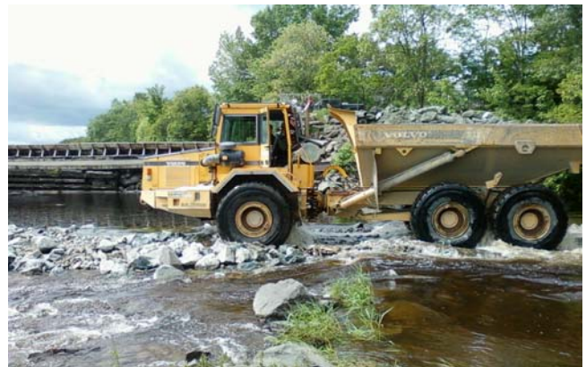
Contractor R.F.Jordan & Sons builds the road out to the dam where removal began June 11, 2012
